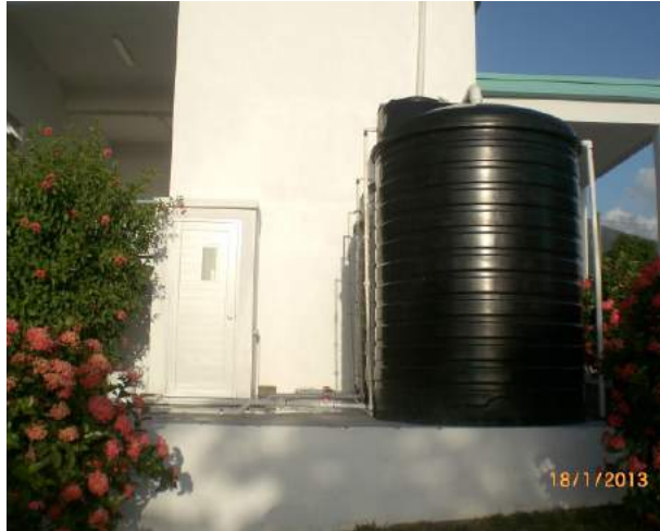
FIGURE 12: NEWLY INSTALLED 1,000 GALLON WATER STORAGE TANK
