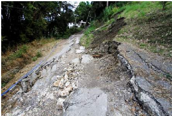
FIGURE 2: LAND SLIPPAGE IN THE SCOTLAND DISTRICT
