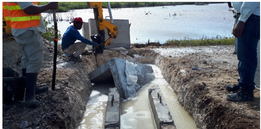
Image 4- Restoration of hydrological flows across a roadway with the use of a culvert at a pilot site for the restoration of mangrove forests in south Clarendon, Jamaica
